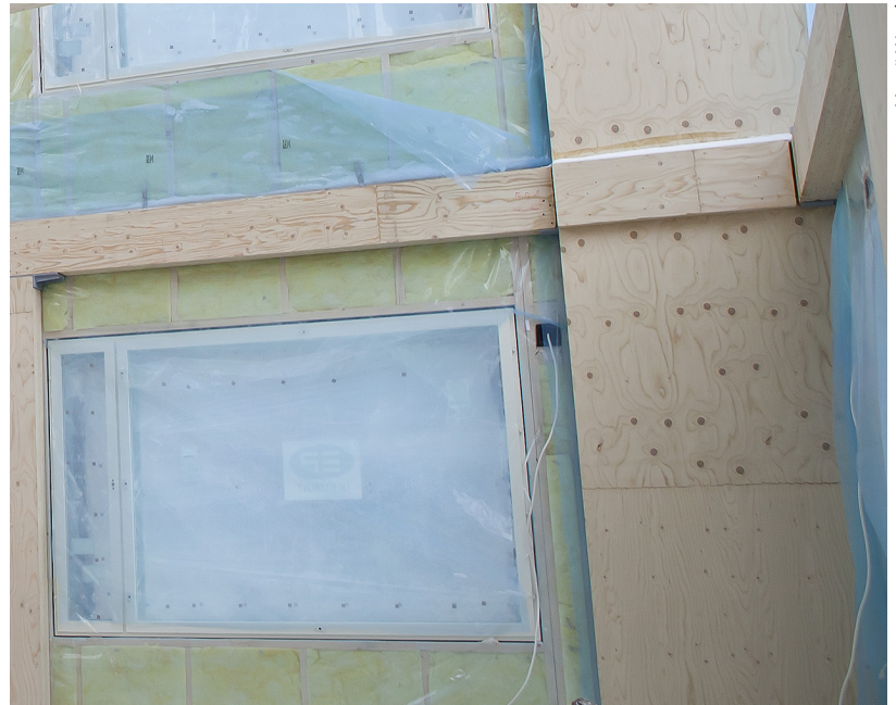
Figure 2.72. LVL-C bracing panels.
