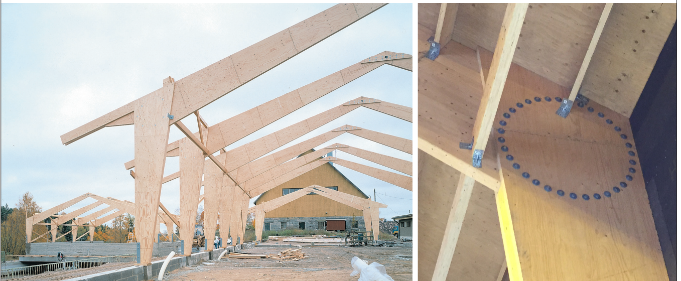
Figure 2.83. 3-pin portal frame structures for hall constructions with moment-resistant bolt circle corner connection.
